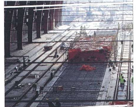
By mid-2003, level +1 of the Central Station will be completed with six operational tracks.
