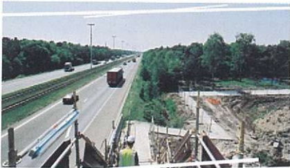
The construction of the high-speed line between Antwerp and the Dutch border started in October 2000. The new railway line will be completed by the end of 2005.
