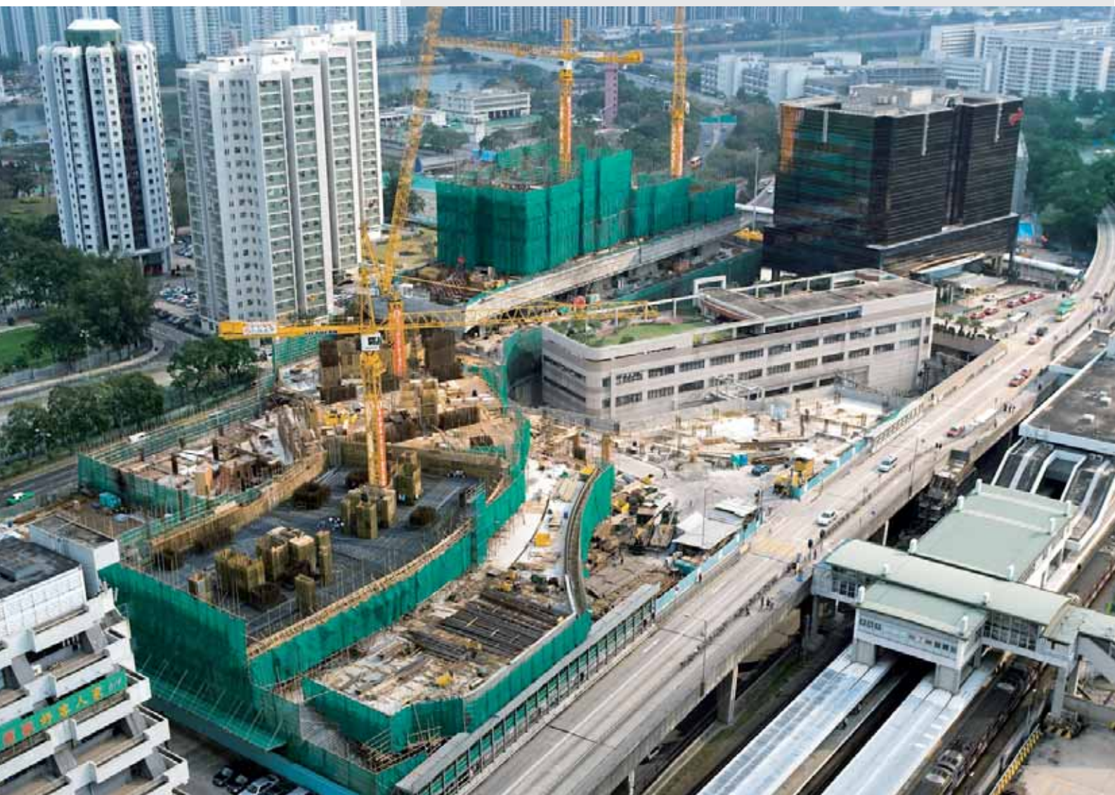
The joint venture development project at Ho Tung Lau (Site A) well underway during the year
