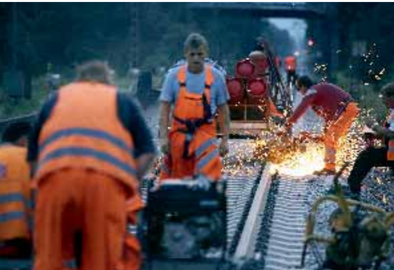
Perfect finish One of the last jobs to be done is the finish grinding of the welded rail heads. Test runs are then made before the line goes back into service.
