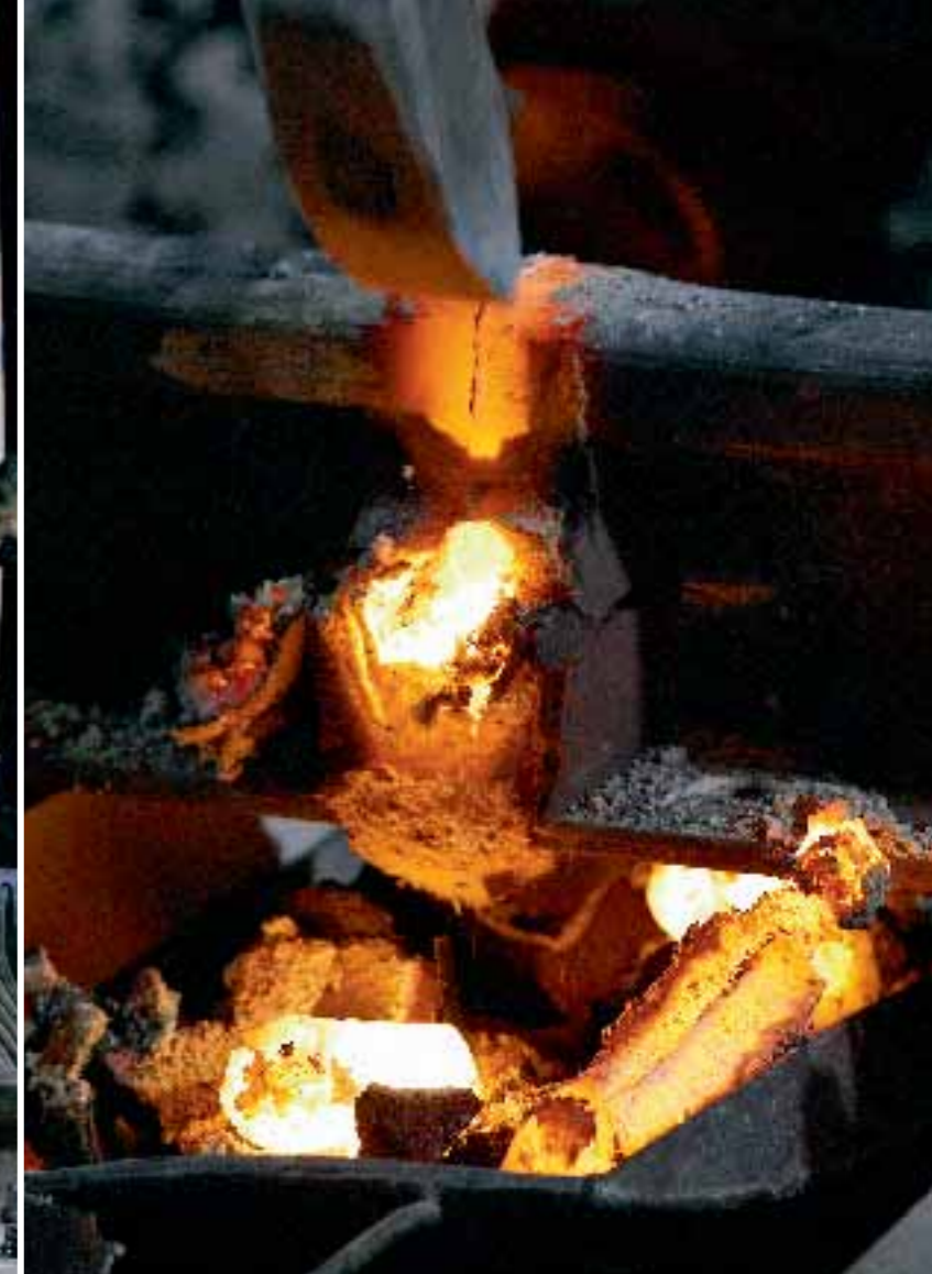
Burn, baby, burn! A highlight for railway enthusiasts is watching rail heads being thermite welded at night. The molten steel at a temperature of 1,000 °C is released into the gap between the rails using welding crucibles.
