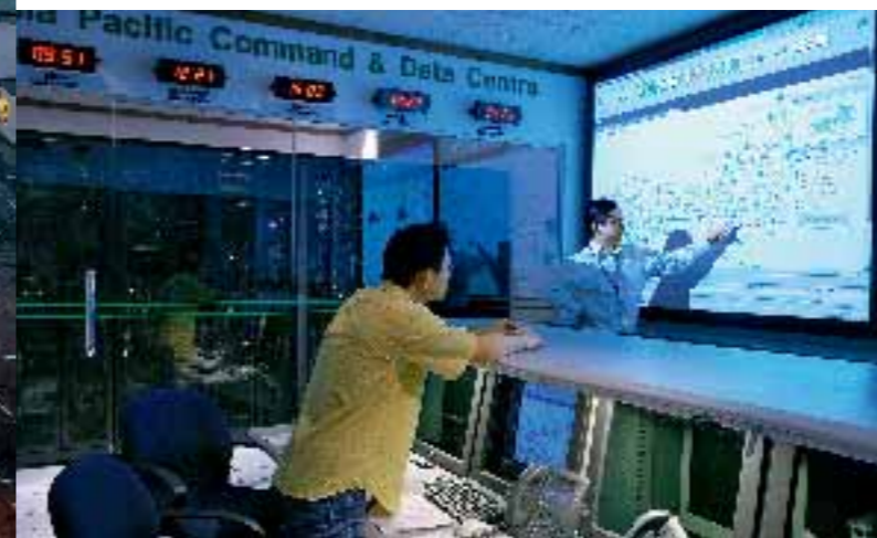
Control panel The scene is Singapore: the Asia Pacific Command & Data Centre monitors and controls the entire IT network structure of DB Schenker's organization in Southeast Asia around the clock and across time zones.
