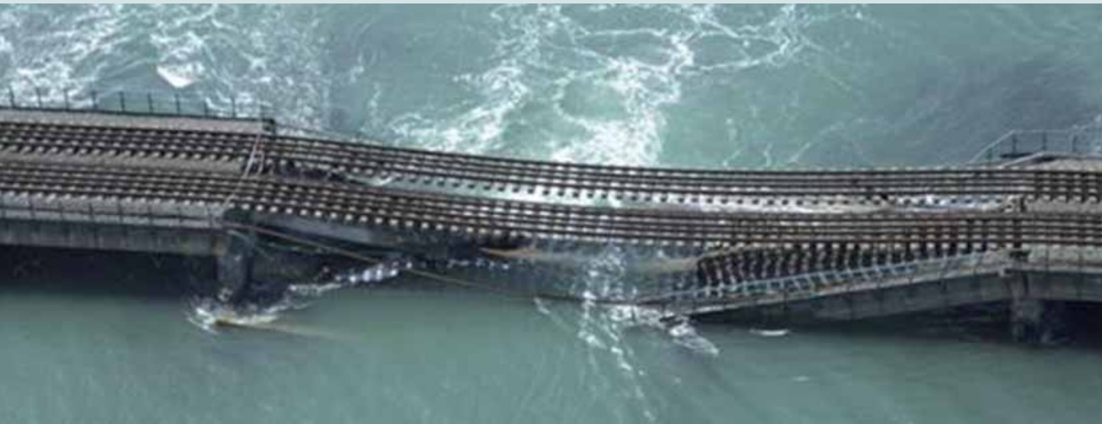
Image 6. Bridge collapse at Malahide, Ireland, 21 August 2009. Photo: Irish NIB
