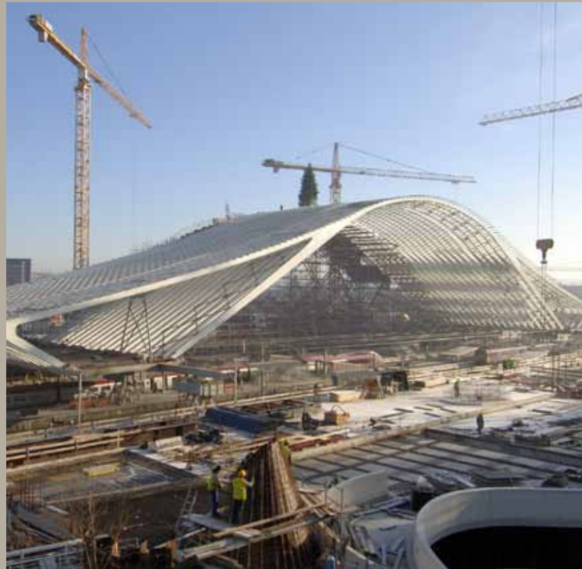
The construction of the vault, pushed over the tracks. One technical exploit calling for another: rail traffic was not interrupted on a single day.
