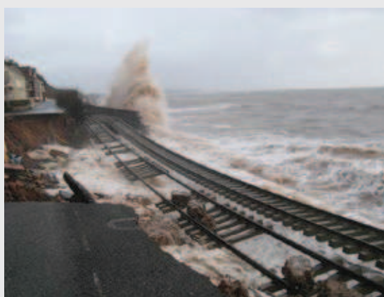
Photo 1.1 Damage to the railway at Dawlish in Devon, the United Kingdom © Network Rail
