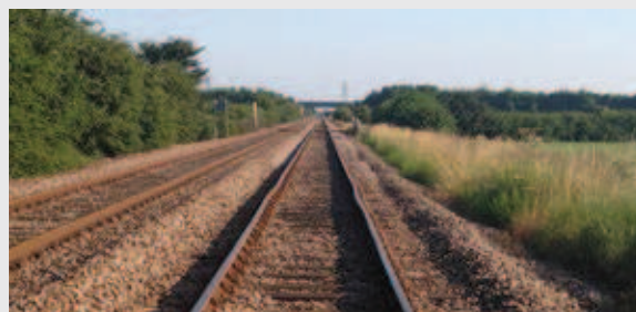
Photo 3.2 Buckled rail © Network Rail
