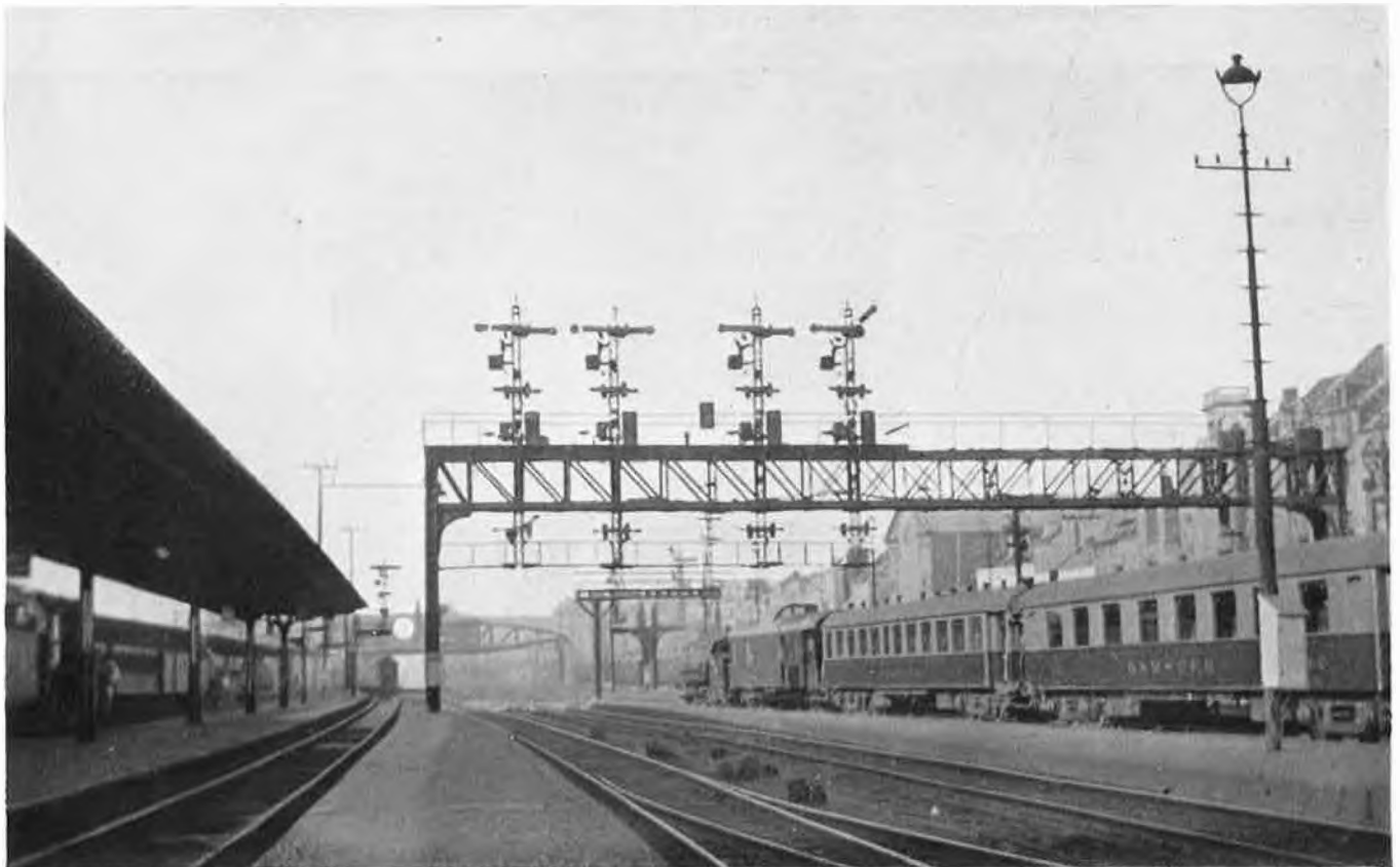
Old Siemens and Halske power signals at Brussels Nord station. The new signal box with electric frame and the recently-installed power-operated points are illustrated on the opposite page. On the right of the above picture is a train of all-steel coaches as described in the article above
