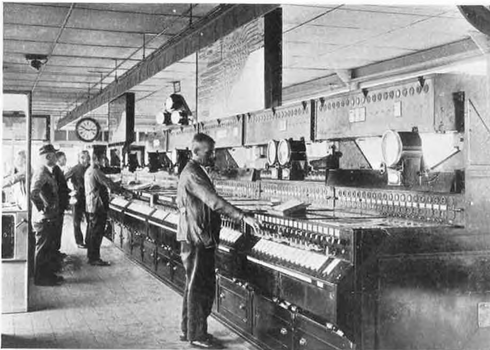
New electric power signal box installed at the Nord station, Brussels, by the Ateliers de Constructions Electriques de Charleroi
