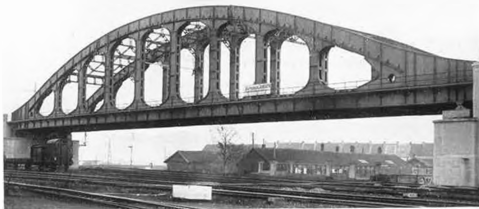
Steel bridge carrying the electric over the steam lines to the north of Malines station, Belgian National Railways
