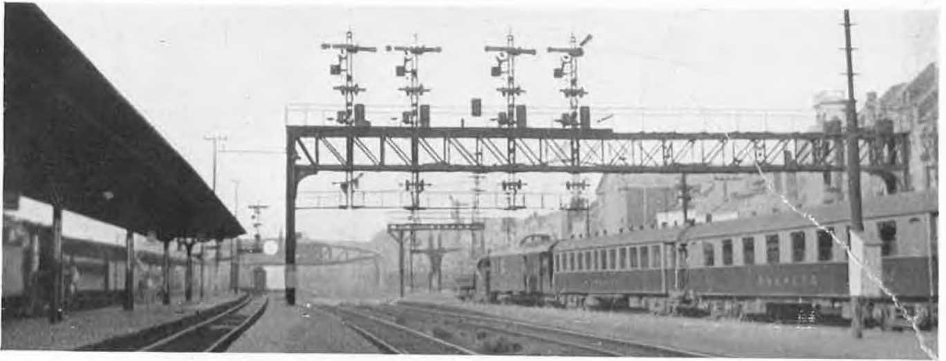
Old Siemens and Halske power signals at Brussels Nord station. On the right of the picture is a train of all-steel coaches
