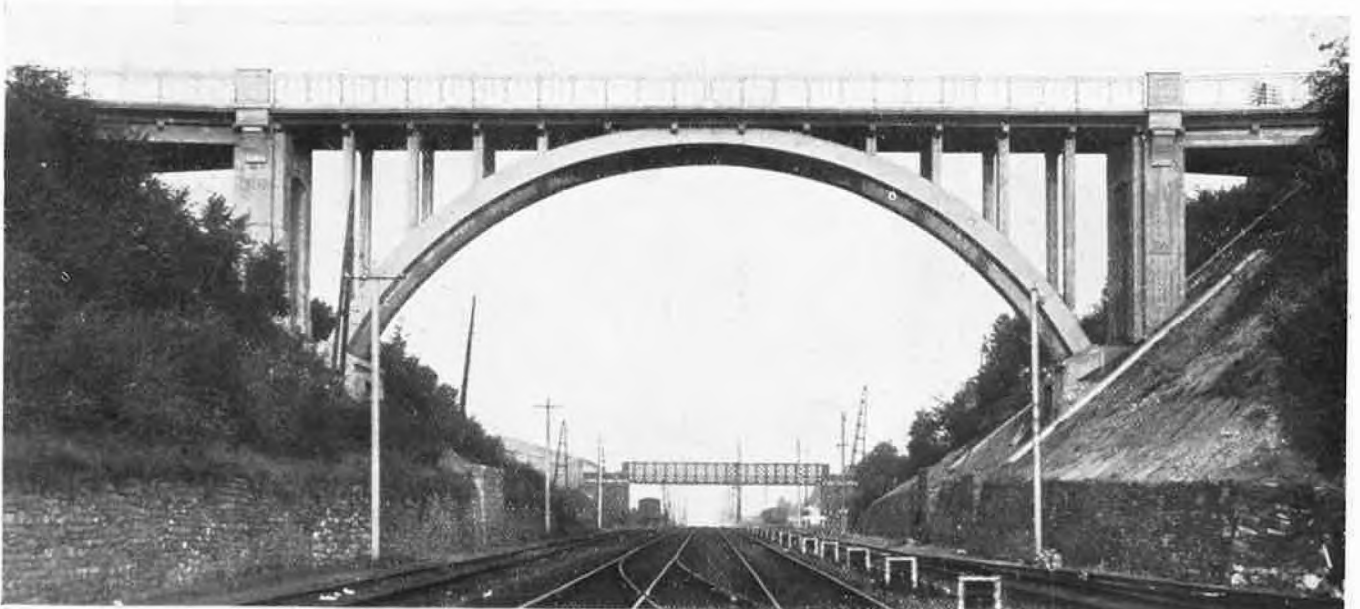
A handsome single span across the Luxembourg line of the Belgian National Railways
